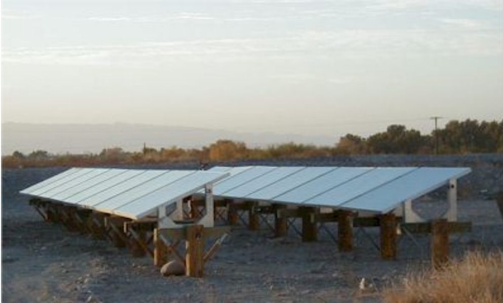
Photo Plate 7: Use of Timber Construction Materials in a Ground-Mounted Solar System
