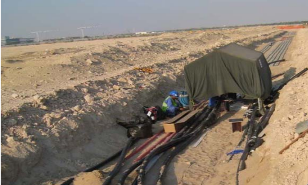
Photo Plate 11: Example of Cabling Being Installed in Trenches for Interconnection to Grid
